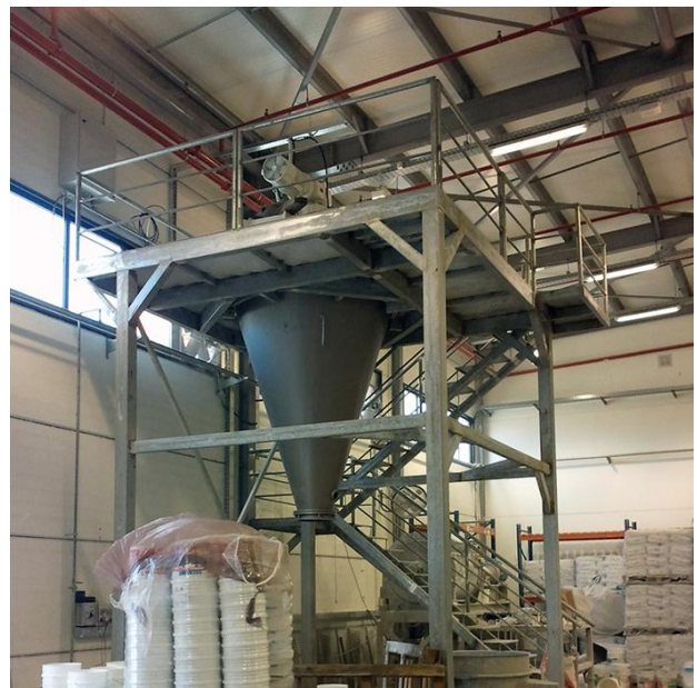
Conical Screw Mixers Installed with Platform
